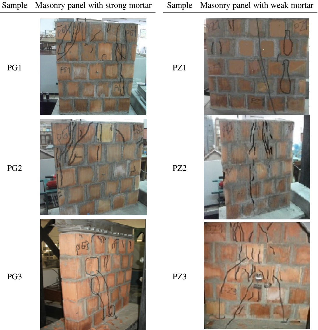
Figure 9. Cracks on the brick masonry panel with M:1.3 (strong) and M:1:6 (weak) mortars after loading.
