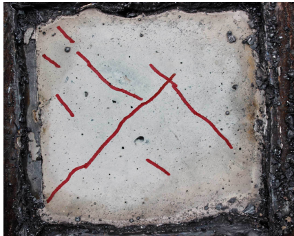
Concrete cracks in early stage
