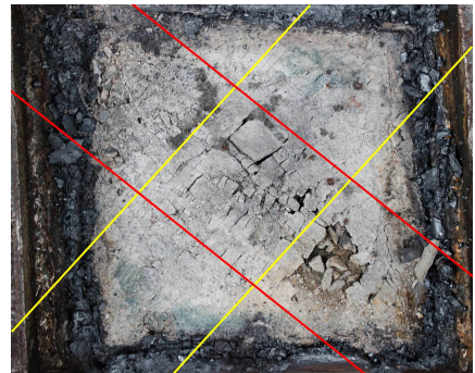
Concrete compression strut crushed
