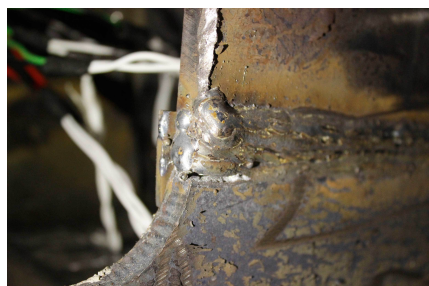
Crack of diaphragm
