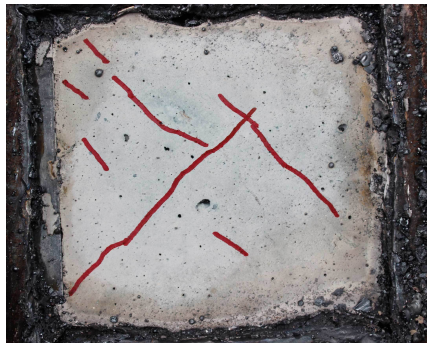
Concrete cracks in early stage
