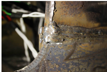
Crack of diaphragm
