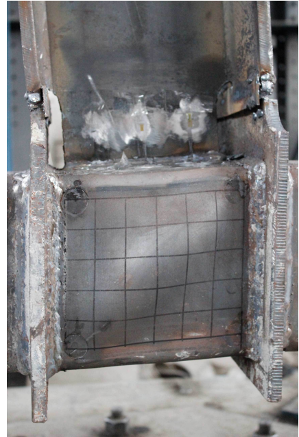
Bulged outward of column web
