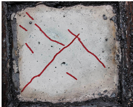
Concrete cracks in early stage
