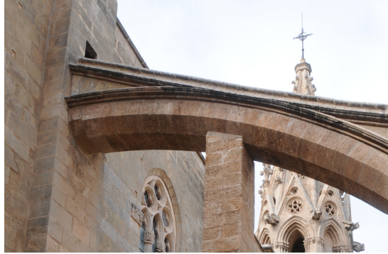
Figure 14. Sliding in the upper flying buttress B6N. Note that the sliding is not between the wall and the first voussoir, but between first and second voussoirs [Photo: Roland Wiczorek, BTU Cottbus-Senftenberg].
