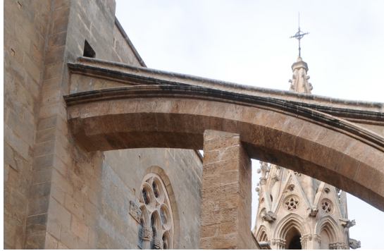
Figure 14. Sliding in the upper flying buttress B6N. Note that the sliding is not between the wall and the first voussoir, but between first and second voussoirs [Photo: Roland Wiczorek, BTU Cottbus-Senftenberg].
