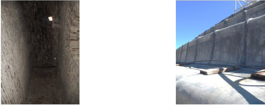
Figure 3. San Francesco di Paola in Naples: particular of the annular aisle in the drum (circled in red in Figure 1 , right), whose structure is made of solid brick walls (left) and view of the upper surface of the dome covered with lead (right).
