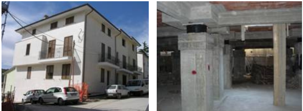
Figure 43. Left: residential building in San Giuliano di Puglia, isolated by 13 HDRBs and 2 SDs with the collaboration of ENEA, completed in 2007. Right: SI formed by LRBs and SDs of an 8-storey building under construction at Messina, in seismic zone 1; its safety will be certified by A. Martelli.
