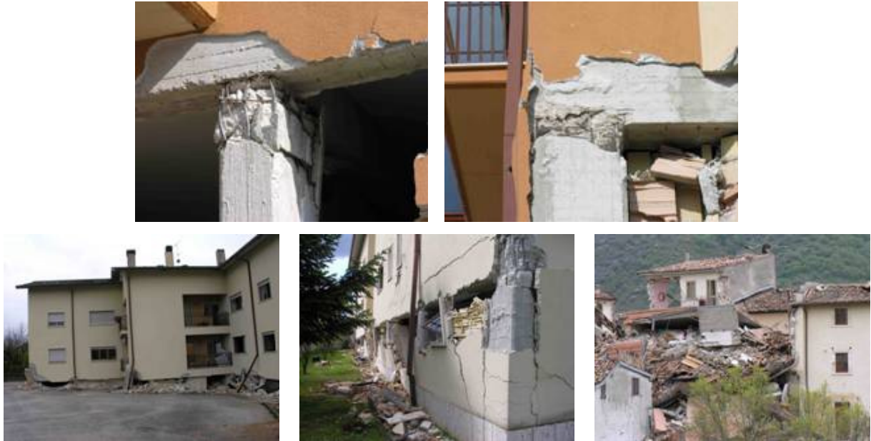
Figure 30. L'Aquila (April 2009): partly collapsed and heavily damaged private buildings. Note in particular the heavily damaged beam-column joints (top row).
