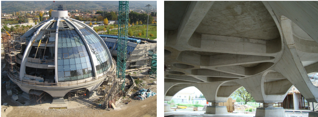
Figure 35. The Emergency and Management Operative Center of the new Civil Defense Center of Central Italy in Foligno (Perugia) was designed by the GLIS board and ASSISi member A. Parducci of e-Campus University. Their safety will soon be certified by A. Martelli. The photo on the left shows in the foreground the main building, which is being erected on ten HDRBs of 1 m diameter, two of which are seen on the right, with provisional protective covers. Also seen on the left is the adjacent service building, isolated by HDRBs and SDs. The Foligno Center will include at least seven isolated buildings, three of which have already been completed. Its site was reclassified from seismic category 2 to seismic zone 1 in 2003, but no design changes of the structures and foundations were necessary, thanks to SI. An increase in the diameters of isolators was sufficient, as demonstrated by a study performed by ENEA.
