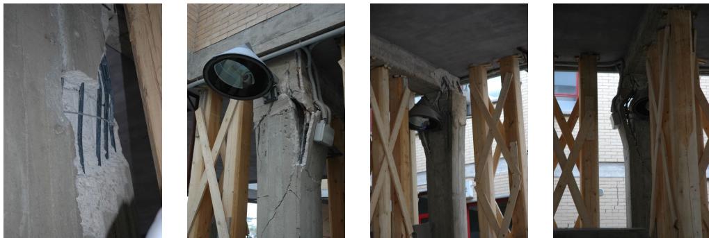
Figure 29. L'Aquila (April 2009): pillars in the San Salvatore Hospital, heavily damaged due to very inadequate steel reinforcement and poor concrete quality (no inert materials are visible in the upper part of the pillar).
