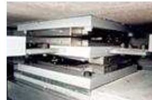
Figure 8. Retrofits with SI in a subfoundation of the National Western Art Museum, designed by Le Corbusier (above), and of the “Gates of Hell” in Tokyo (right column), performed in 1999.
