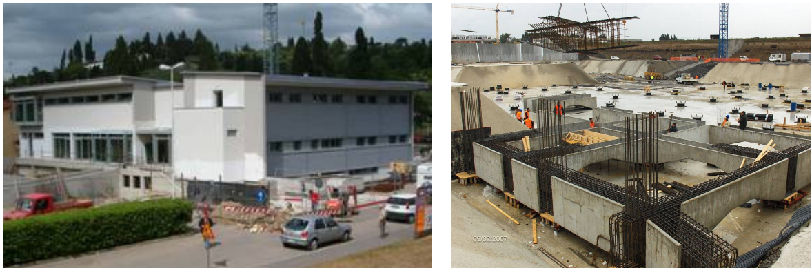
Figure 41. Left: Headquarters of the association Fratellanza Popolare – Croce d’Oro in Grassina (Florence), in seismic zone 2, isolated by means of SDs and VDs; it is a L-shaped building to be used for civil defense, designed by the GLIS board and ASSISi member S. Sorace of the University of Udine and certified as safe by A. Martelli in 2007. Right: NATO Centre in South Naples, in seismic zone 2 (399 HDRBs and 20 dissipative SDs), during construction in 2007.
