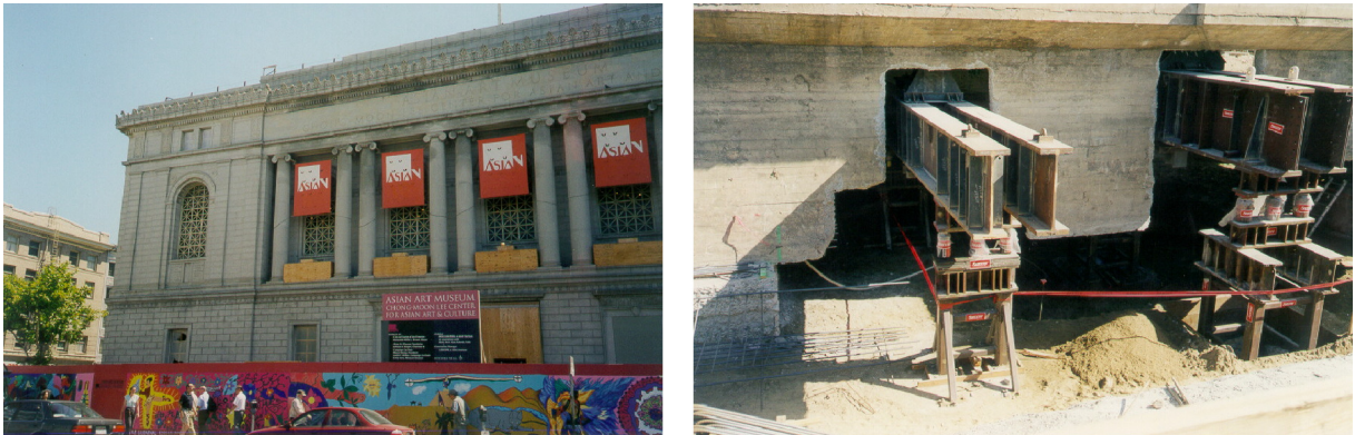
Figure 21. Asian Art Museum in San Francisco, during its seismic retrofit (with cut of the foundations and insertion of HDRBs) performed according to the design of the Italian architect Gae Aulenti (late 1990s).
