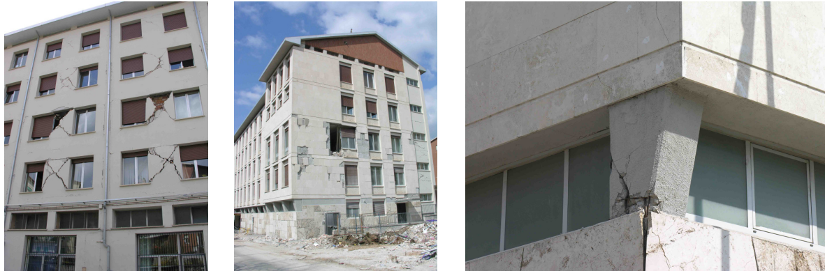
Figure 32. L'Aquila (April 2009): headquarters of ANAS (the Italian agency for road construction and maintenance), which suffered mainly nonstructural damage (with the exception of two pillars, which, however, are reparable — see right. Retrofit by means of SI was possible and was suggested for this building.
