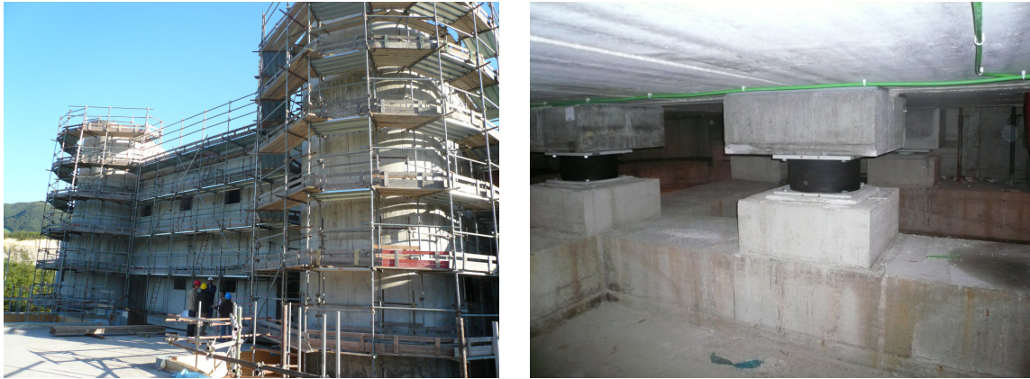
Figure 38. The new school in Marzabotto (Bologna), in seismic zone 3, erected on HDRBs and SDs. Its safety was certified by A. Martelli in September 2010.
