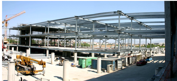
Figure 60. The Shakolas Park Commercial Centre at Nicosia (Cyprus), designed by the Italian GLIS board and ASSISi member G. C. Giuliani and his son of Redesco (Milan), formed by two buildings with mixed r.c. and steel structure, with 164 Italian HDRBs installed at top of the basement columns, during construction in 2007.
