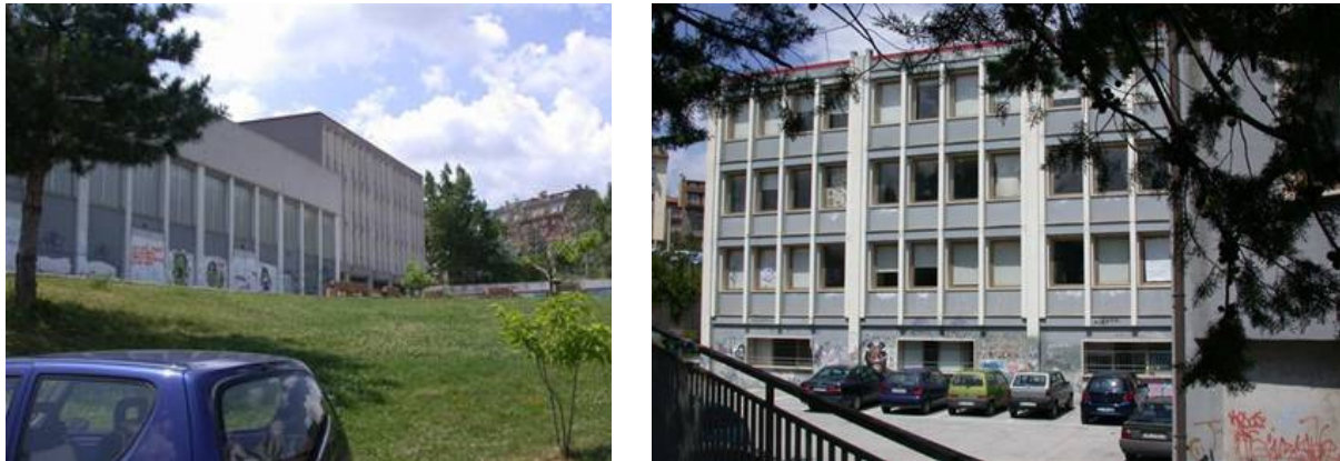
Figure 39. Romita High School for scientific studies of Campobasso (hosting about 1,300 students), in seismic zone 2, which was at last partly demolished and is now being rebuilt with SI, due to its very poor concrete quality (as demonstrated by an ENEA study performed after the 2002 Molise and Puglia earthquake). Safety of the new seismically isolated buildings will be certified by A. Martelli.
