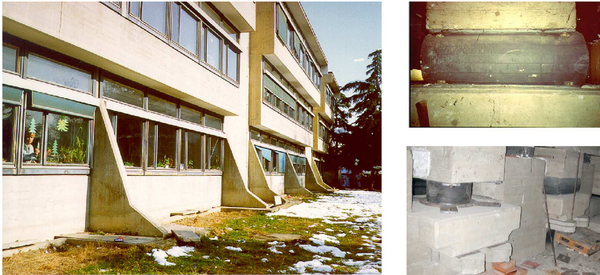
Figure 65. Left: the isolated Pestalozzi school at Skopje (Macedonia), built in the 1960s. Top right: a very degraded original low damping rubber bearing (LDRB). Bottom right: a new HDRB, next to original LDRBs yet to be replaced.
