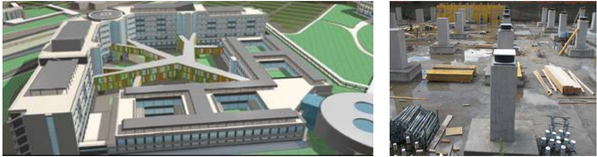
Figure 34. Sketch of the new isolated Del Mare Hospital, during its construction in Naples, nowadays in seismic zone 2, and view of some of its 327 HDRBs. Several new Italian hospitals being or to be erected in seismic areas now include the use of SI.
