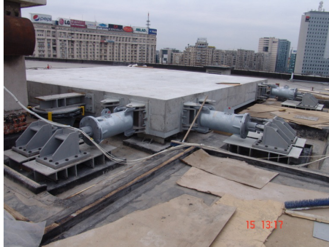
Figure 29. TMCS at roof of building.
