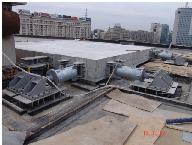
Figure 29. TMCS at roof of building.
