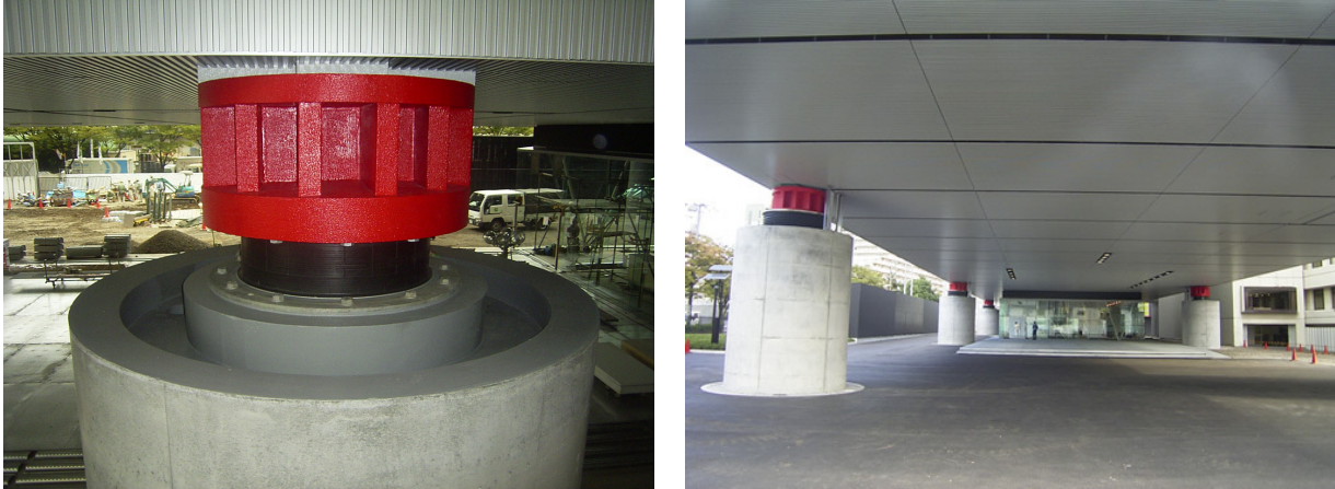
Figure 5. Seismic isolators (lead rubber bearings) on top of first-floor pilotis in the Main Building.
