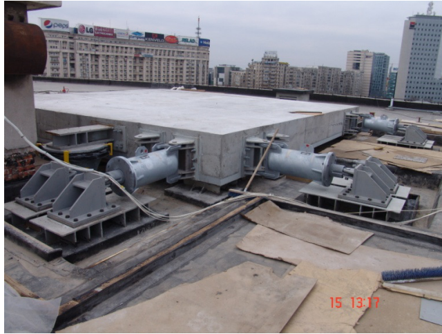
Figure 29. TMCS at roof of building.
